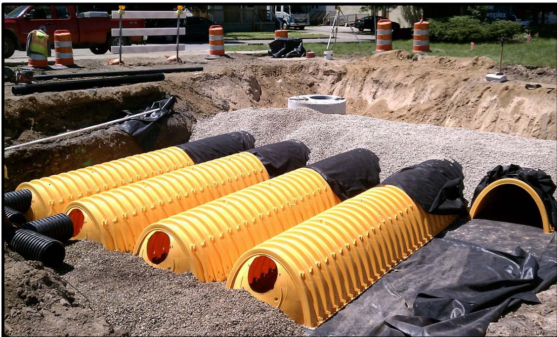
Underground Storage Vault for Water Management
